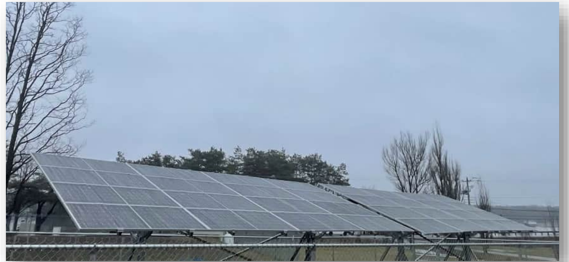
Conquerall Bank ground mount 15 kW solar array
