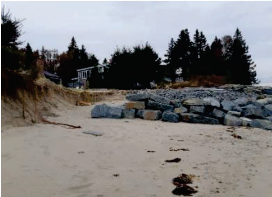
Waves went in behind the armored wall removed sand, and compromised the wall.
