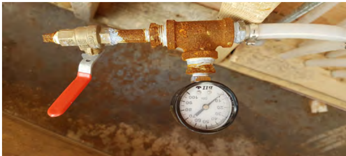
Photo #3 - In-floor Hot Water Heating Piping (pressure gauge reading zero)
