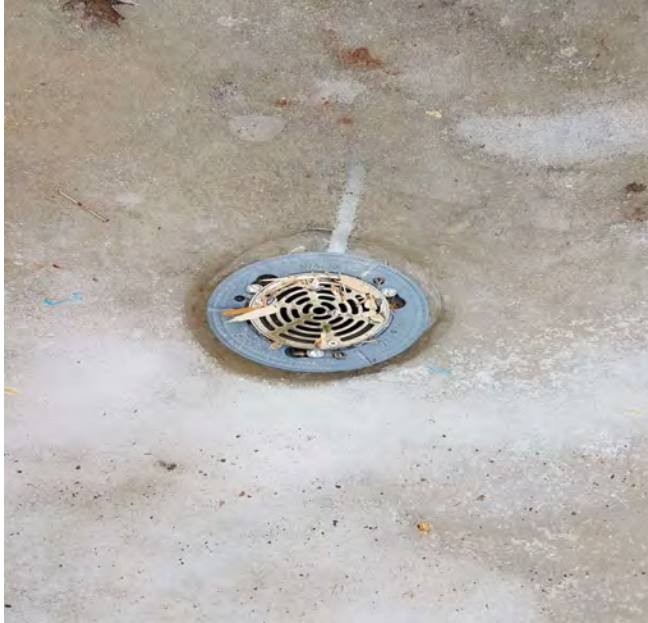
Photo #4 – Floor Drain in Main Entrance (not protected/covered)
