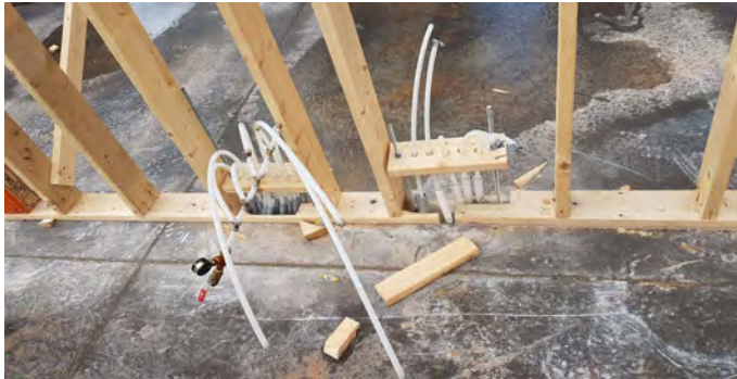
Photo #2 - In-floor Hot Water Heating Piping (not capped yet; no pressure test)
