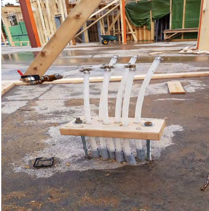
Photo #1 - In-floor Hot Water Heating Piping c/w Pressure Test Gauge and Pipe Sleeves
