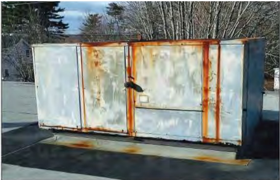
Original Lennox Rooftop Unit
