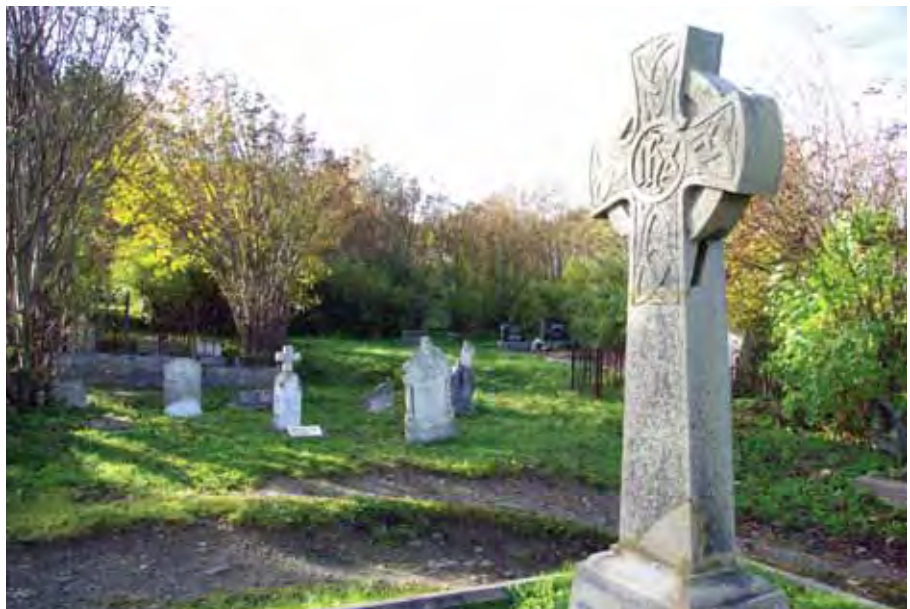
A condition assessment and evaluation undertaken before an intervention at Belvedere Cemetery in St. John's Ecclesiastical District, would reveal that the well-aged and weathered patina found on the grave markers is not damaging. It is in fact a character-defining element of this historic place and should be preserved.
