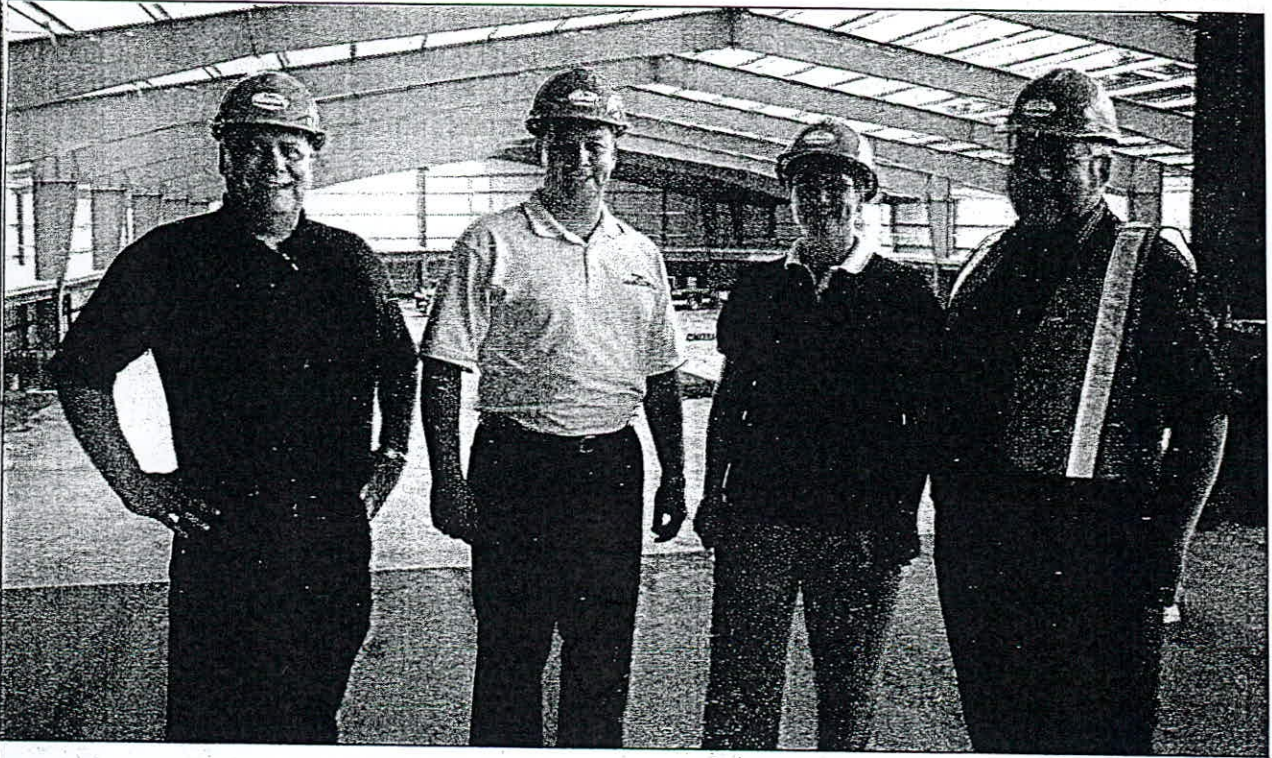
Scott Patterson and Doug Quinn, members of the South Shore Fieldhouse Society, took the Premier and MLA Carolyn Bolivar-Getson on a tour of the facility under construction. The MacDonald government contributed $898,000 towards construction of the fieldhouse.
