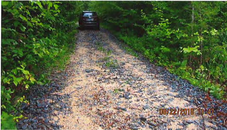
Private park upper driveway in need of widening. (Source: EDM)
