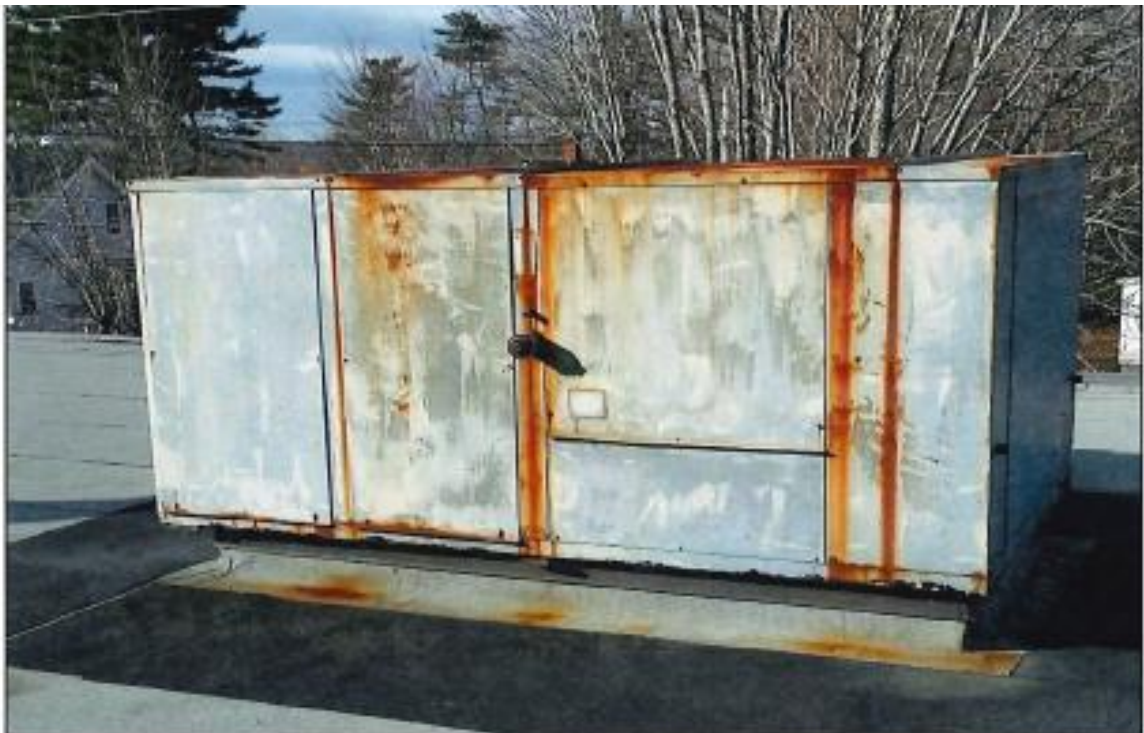
Original Lennox Rooftop Unit
