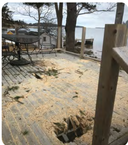
Shoreline property showing debris, sediment, and damage on a deck or waterfront area following high water or storm conditions.
