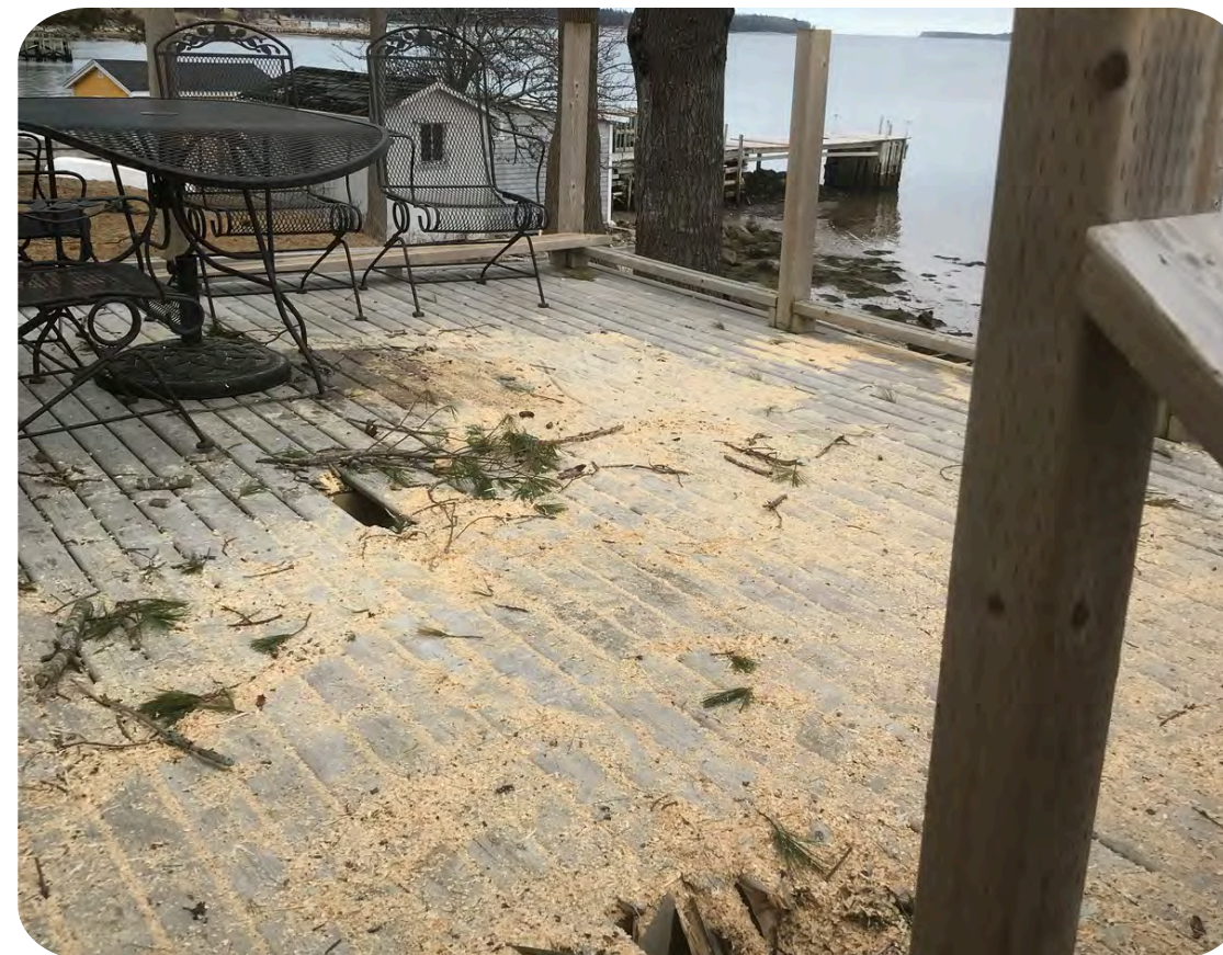
Shoreline property showing debris, sediment, and damage on a deck or waterfront area following high water or storm conditions.
