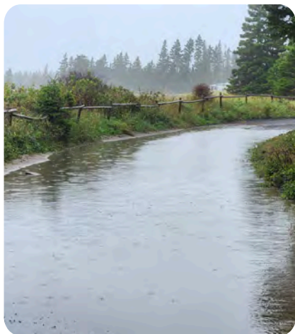
Roadway flooding following heavy rainfall, showing water covering the road surface and affecting access.
