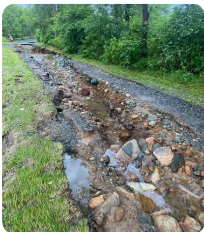
Washed-out roadway or driveway showing exposed rocks and erosion following heavy rainfall or flooding.
