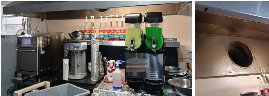
Picture 1 – Existing Range Hood
